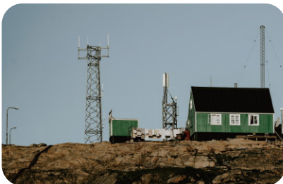
5G Communication Base Station
