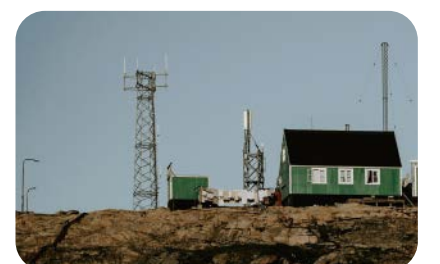
5G Communication Base Station
